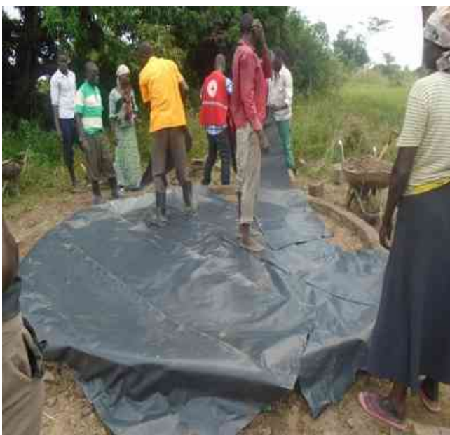
CBDRR member and the community members construct the foundation of a flood-resistant hut. Photo: URCS
